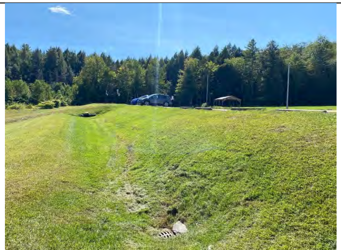
Photo 2: Swale along east side of parking lot that does not receive runoff due to poor site grading
